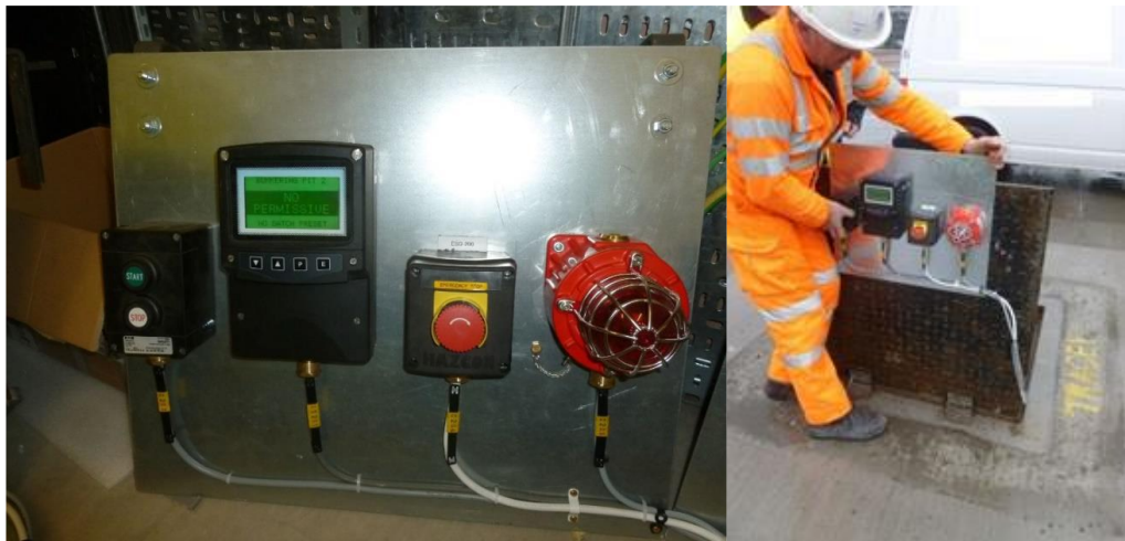
Figure 4-1 Typical Bunkering Point Control Equipment
