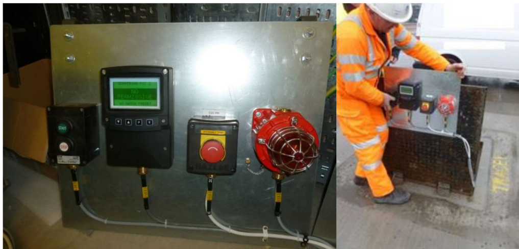
Figure 4-1 Typical Bunkering Point Control Equipment
